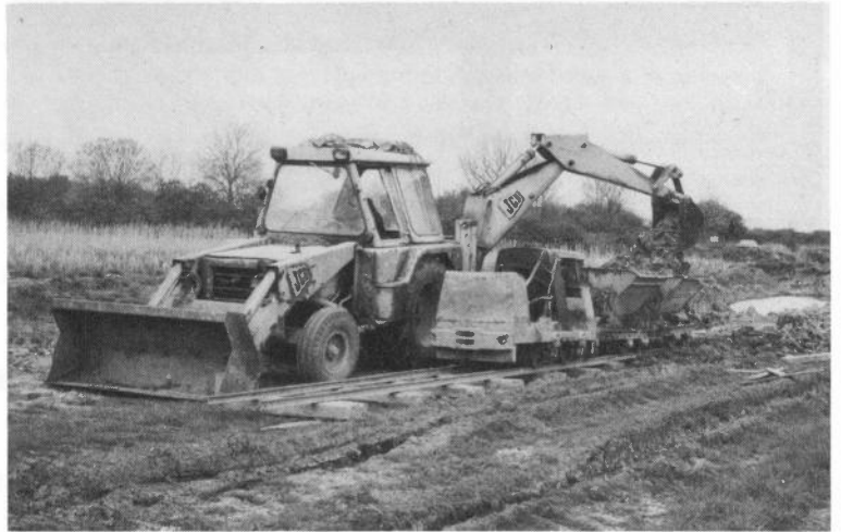
Ruston & Hornsby 247182 stands alongside the JCB digger which loads clay into the two skips. (A.J. Booth)
